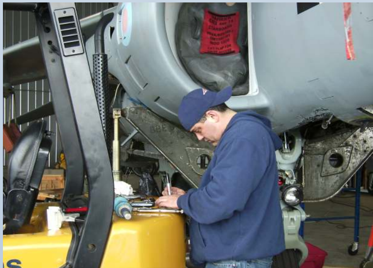
Christian Vlahos is laying out one of several repairs to the inner structure. The forklift is an excellent workbench.
